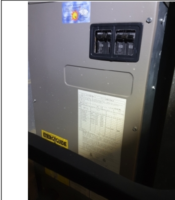
Shut off switches
