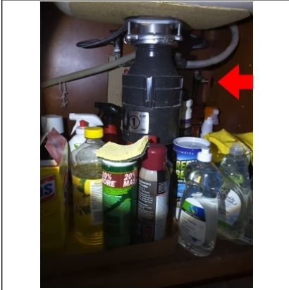
Shut off valves
