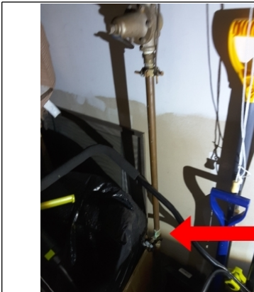
Main supply valve basement
